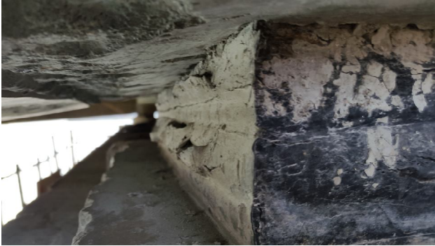
Figure 6. Condition of a typical bearing
