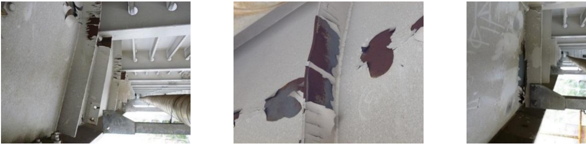
(a) (b) (c) Figure 5. Damages due to collision (a) Bent transverse-stiffeners and strut separated from stiffener (b) Buckled transverse-stiffener (c) Transverse stiffener separated from web.
