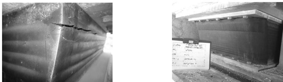
(a) Ozone cracks appearing on a poor quality rubber bearing (b) Bearing after 5 years of treatment using K-Coat-R
